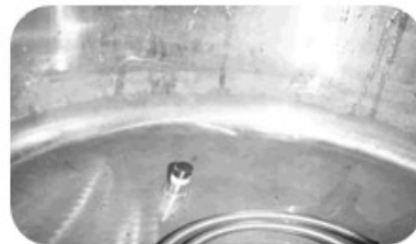
Water level sensor
